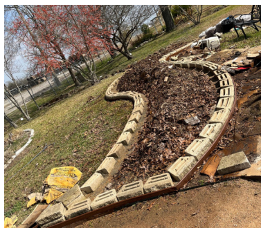
The pavers are set in quikrete for stability in maintaining the design.
